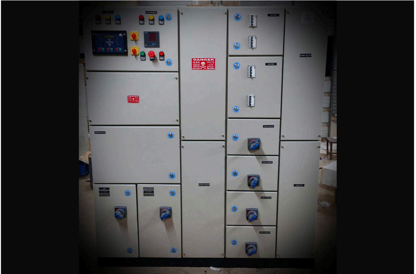
Complete AMF / ATS Panel Board — KSEB & Diesel Generator Incomer with Full Distribution
